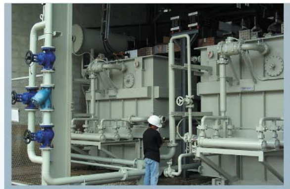
■ 4921/2 x 3480 kVA 22000 - 200 VAC Padaeng Industries Public Company Limited
